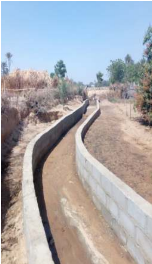
CONSTRUCTION OF DRAINAGES AND CULVERTS AT GALAMAWA QUARTERS, DUTSE LOCAL GOVERNMENT AREA
