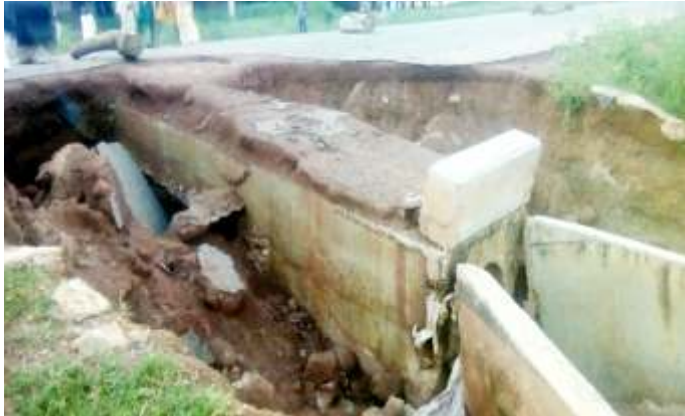
FAILED SECTION OF GADAMA CULVERTS (NO.1) ON GWARAM- FAGAM ROAD
