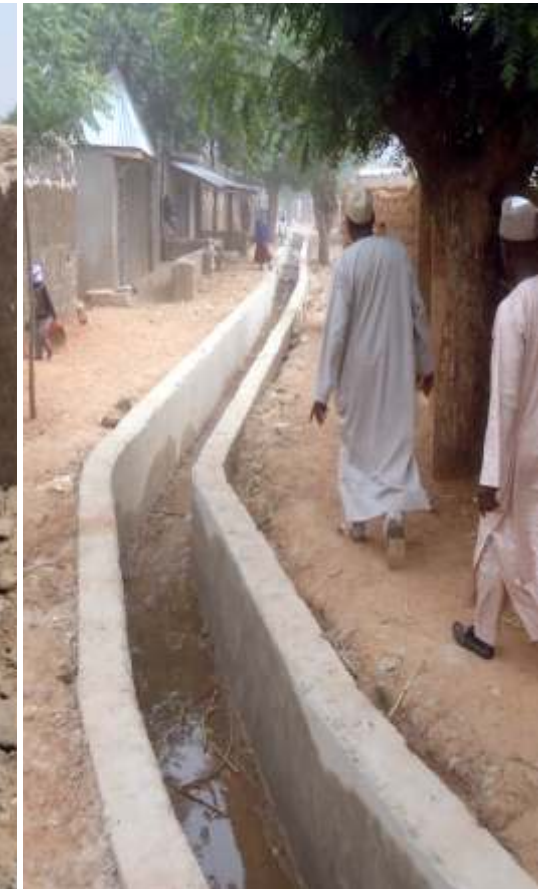
CONSTRUCTION OF DRAINAGES AND CULVERTS AT LIMAWA QUARTERS, DUTSE LOCAL GOVERNMENT AREA
