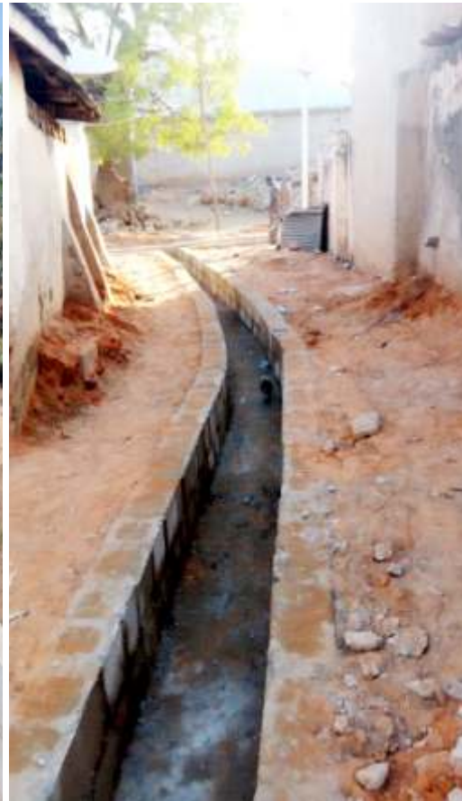
CONSTRUCTION OF DRAINAGES AND CULVERTS AT GARU DUTSE QUARTERS, DUTSE LOCAL GOVERNMENT AREA
