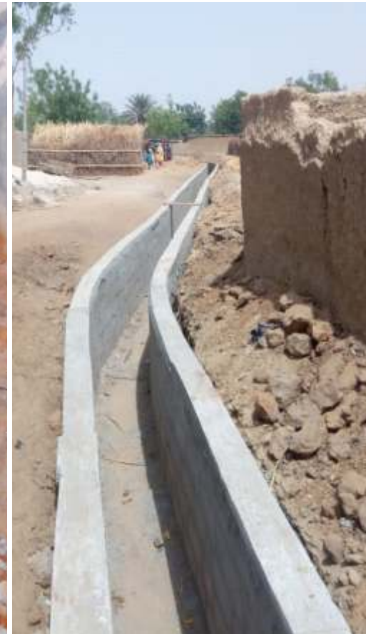
CONSTRUCTION OF DRAINAGES AND CULVERTS AT CHAMO TOWN, DUTSE LOCAL GOVERNMENT AREA
