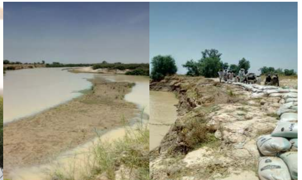
River embankment at Malamawar, Taura
