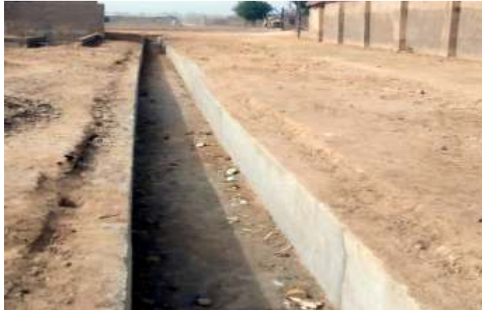
CONSTRUCTION OF DRAINAGES AND CULVERTS AT SABON GARI QUARTERS, BIRNIN KUDU TOWN, BIRNIN KUDU LOCAL GOVERNMENT AREA
