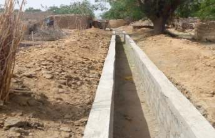
CONSTRUCTION OF DRAINAGES AND CULVERTS AT CHAMO TOWN, DUTSE LOCAL GOVERNMENT AREA
