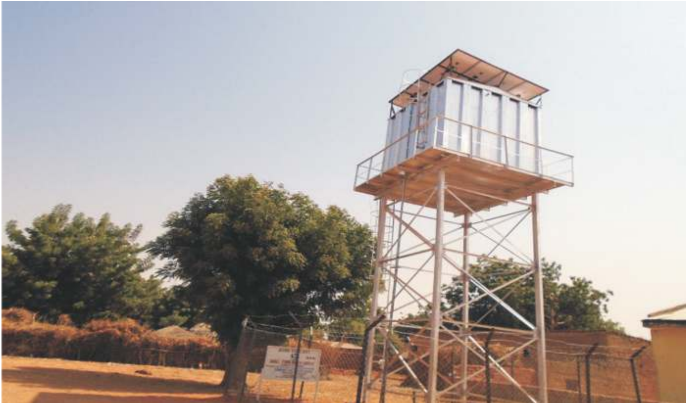
One of the newly constructed Solar Powered water supply scheme at Sabaru town in Kazaure LGA (Constituency)
