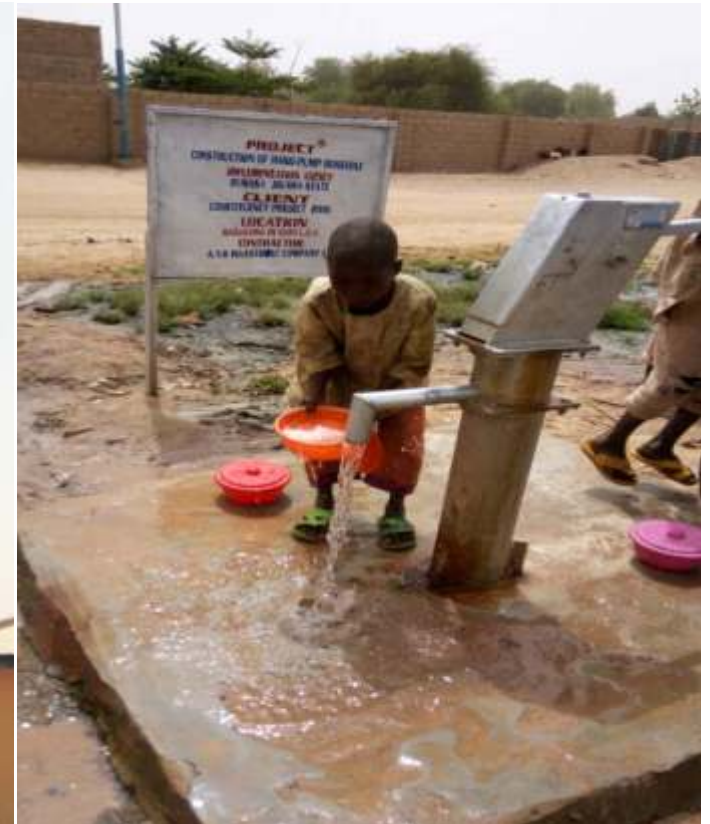
One of the newly constructed hand pump borehole in Nasarawa Guri LGA
