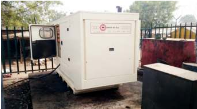
NEW 100 KVA GENSET AT KIYAWA MOSQUE
